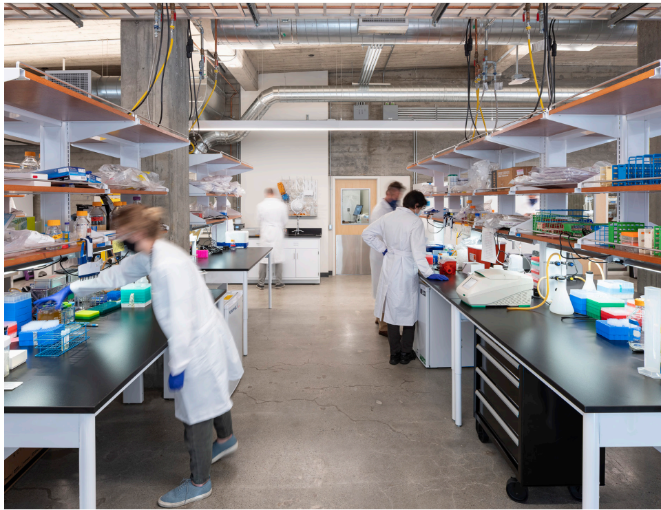
Ceiling service panels (CSPs) located on a modular basis to benches
